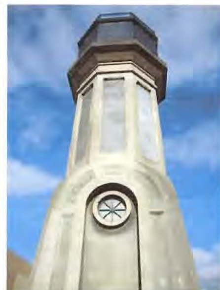
Addington Water Tower with some damage from the February 2011 Christchurch earthquake
